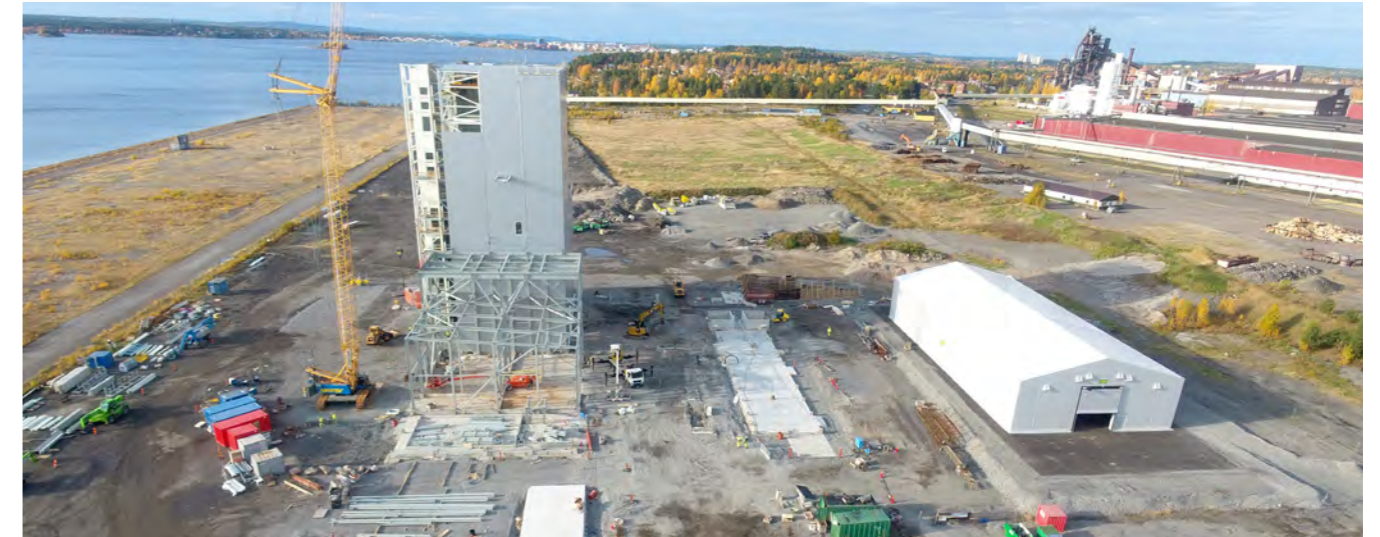
The Hybrit project explores the possibility of fossil-free steel production by replacing the carbon currently used in the process with hydrogen. Image Credit: HYBRIT
